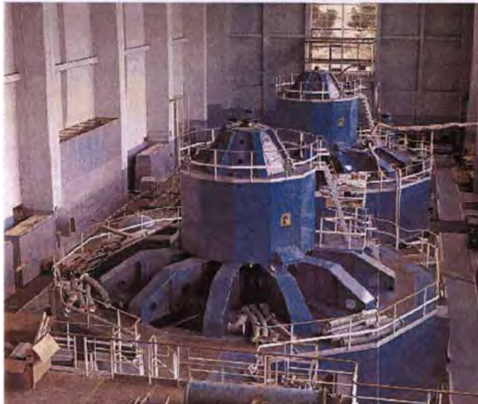
Turbine hall of the Eildon Power Station.
