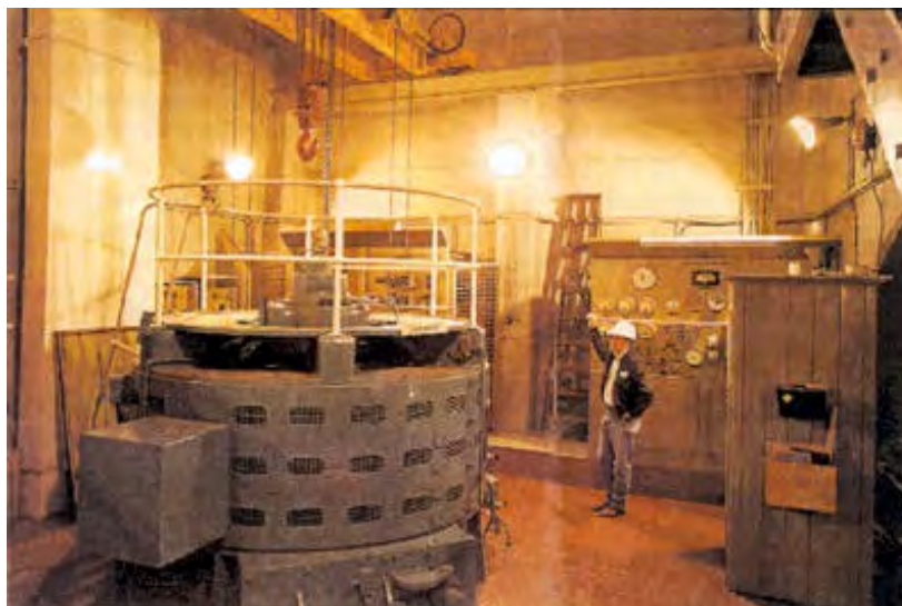
Cairn Curran power station generator room.
