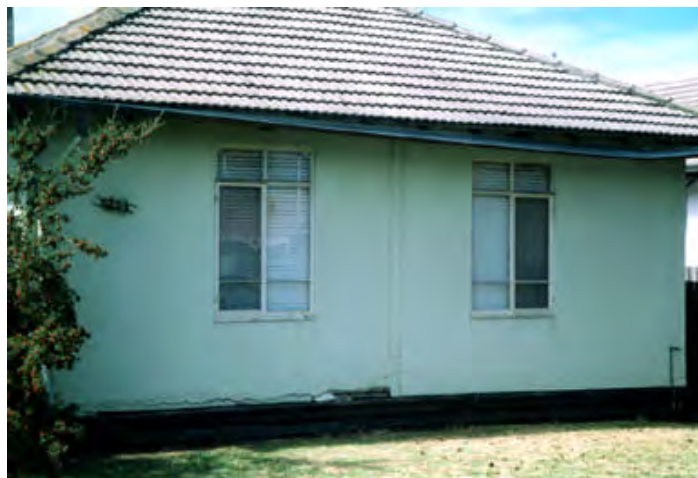
An example of repairs required to roof guttering.
