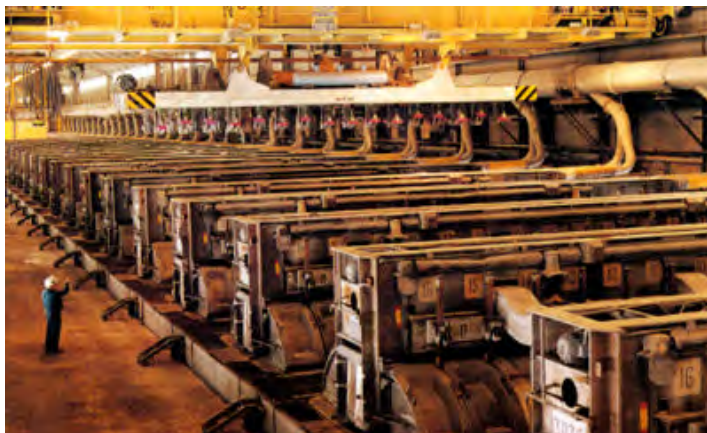
One of 4 pot-rooms at the Portland Smelter. (Photo courtesy of ALUVIC.)
