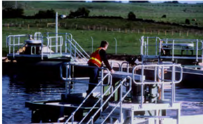
Upgraded facilities at the Portland Coast Region Water Authority wastewater treatment plant.
