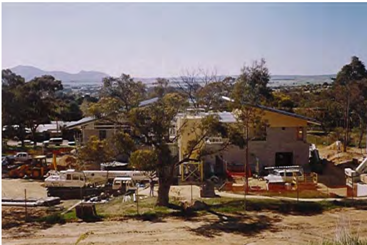
Commencement of the construction of the water treatment facility at Halls Gap. (Photo courtesy of the Grampians Region Water Authority.)
