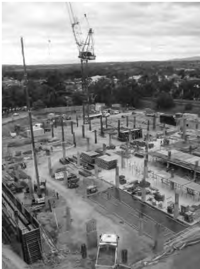
Car park construction works on the Austin site. (Source: ARM Project team.)
