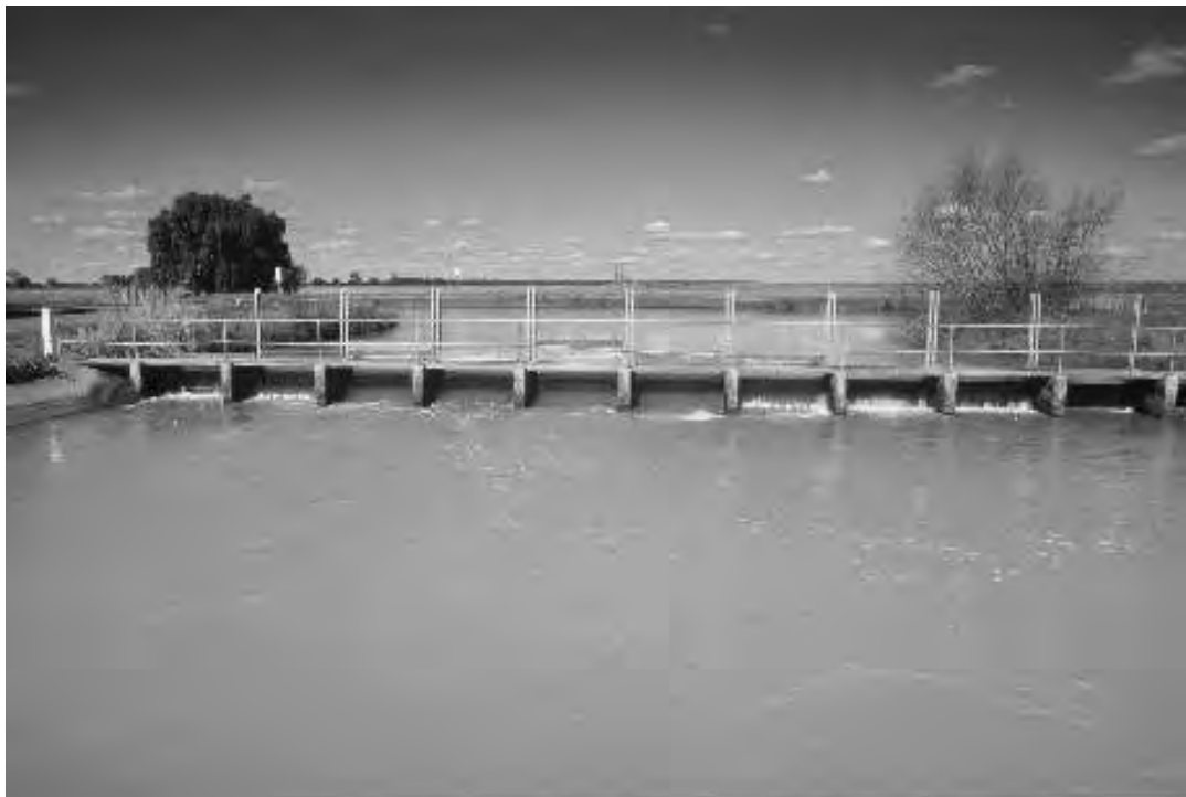
Regulator minor outlet at Waranga basin.
