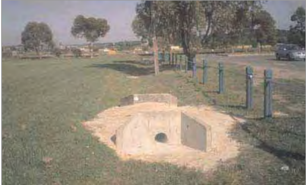
Jack Thomas Reserve - Casey constructed culverts and installed them in existing opens drains.
