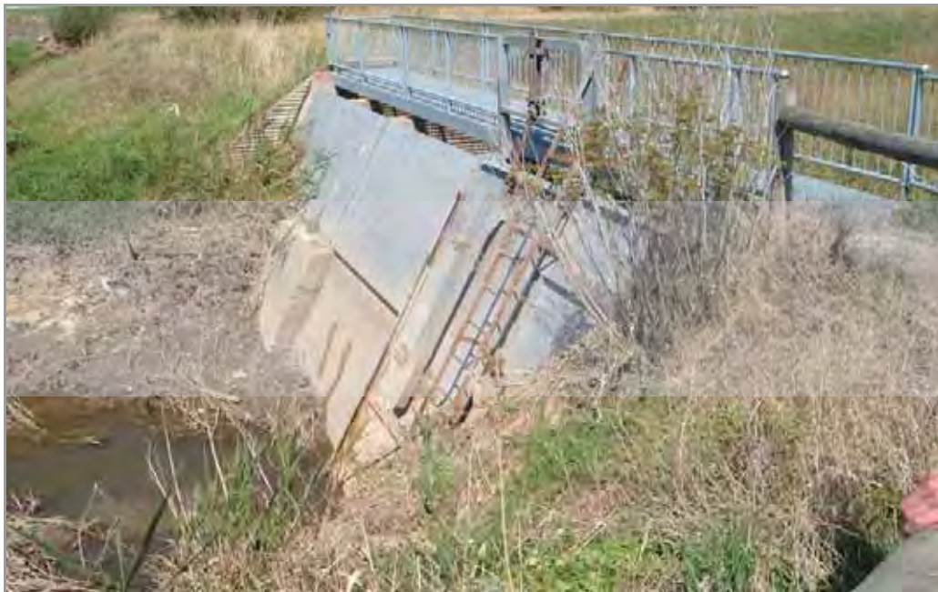
A Melbourne Water stormwater drainage asset to control water flow along a creek.
