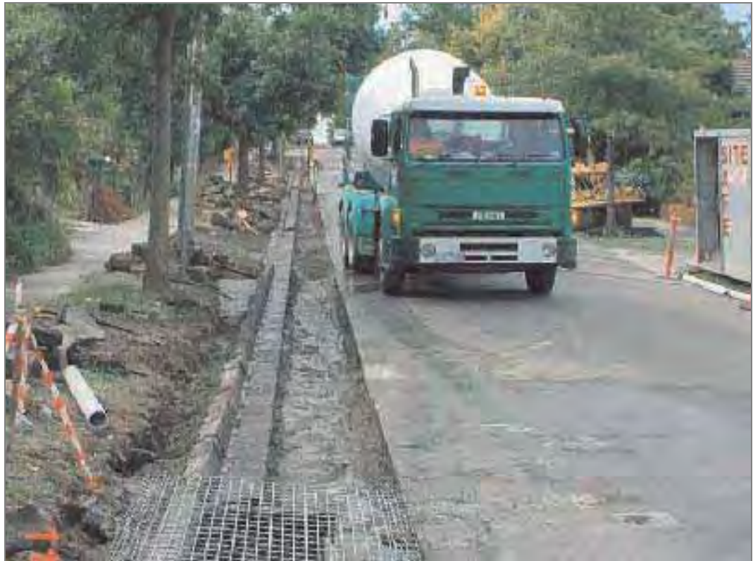
Boroondara constructed a new pit with a grated cover, widening 2 pits and upgrading the drain from a semi-circular brick drain to a 525 mm diameter concrete pipe.
