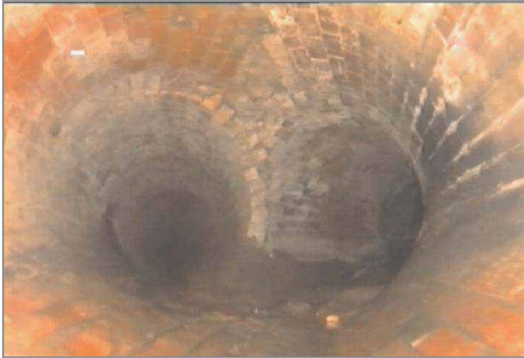
Boroondara closed circuit television condition assessment of brick drain, Auburn Road, Hawthorn.
