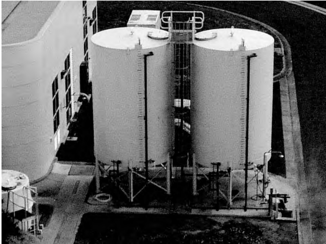
PAC23 chemical storage tanks at the Wurdee-Boluc water treatment plant, from which one of the chemical samples was taken for testing.
