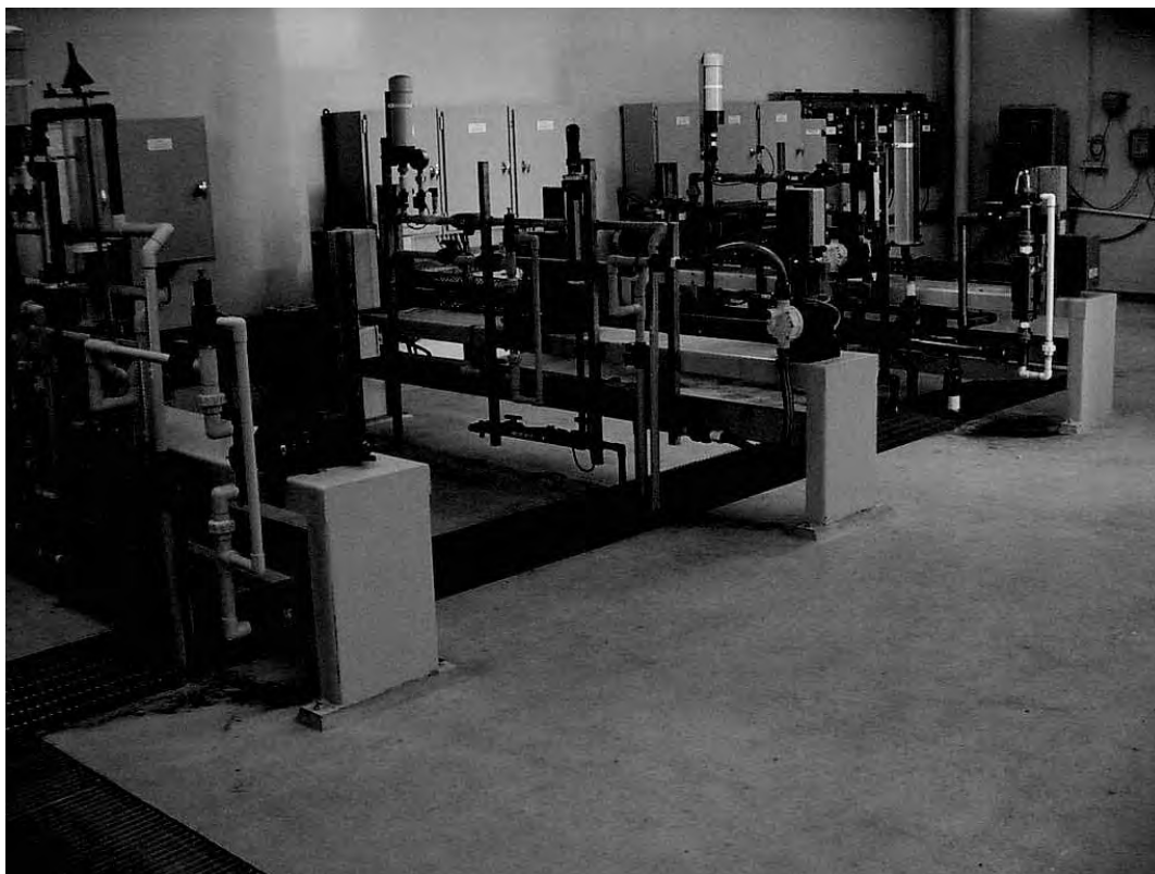
Computerised equipment in use in the water treatment process at the Wurdee-Boluc water treatment plant. The efficient function of such equipment is at risk if poor quality chemicals are used in the treatment process.
