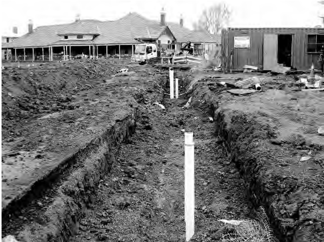
New services and utilities being installed in the heritage precinct. (Photo courtesy of Major Projects Victoria.)
