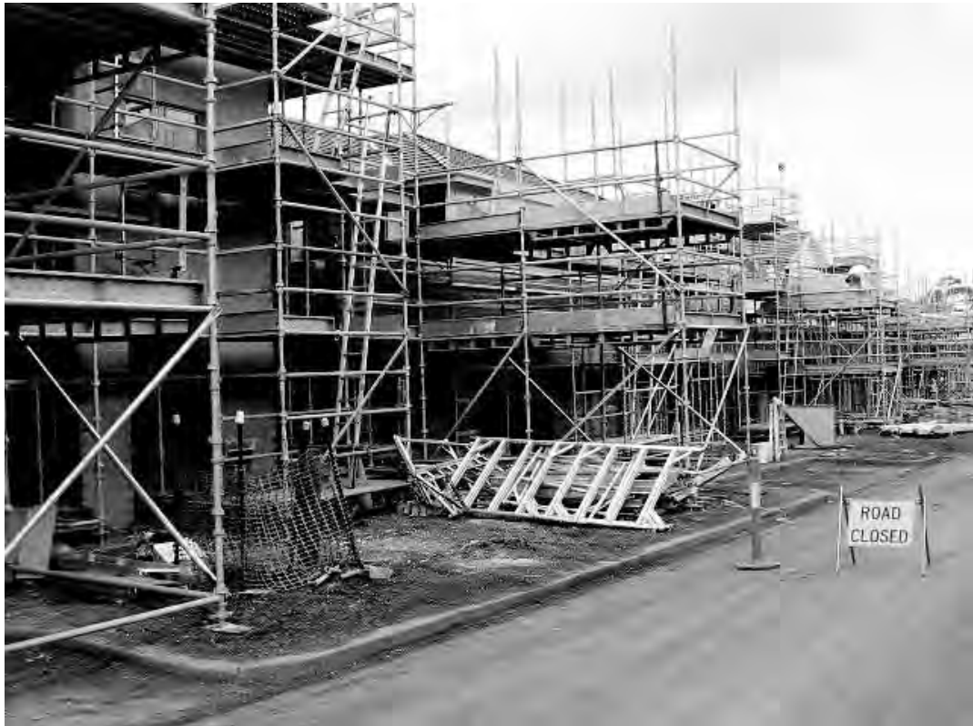
Houses under construction in the athletes' village. (Photo courtesy of Major Projects Victoria.)
