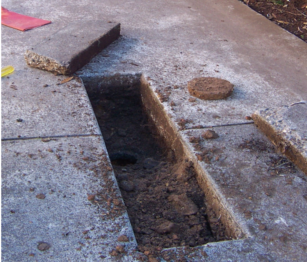
Septic tank situated beneath a concrete driveway. Property owners sometimes make alterations to their homes that render septic tank maintenance and monitoring difficult, if not impossible. (Photo courtesy of Ballarat City Council.)
