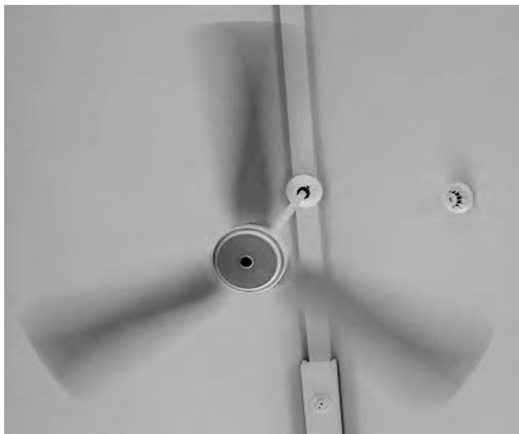
Placement of smoke detector too close to ceiling fan reduces the detector's effectiveness.
