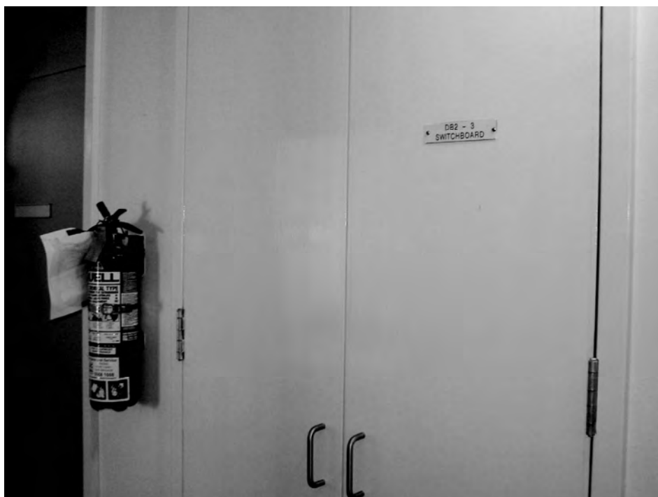
Fire extinguisher located within 2 metres of electrical switchboard.
