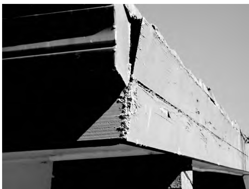
Fascia in poor condition.
