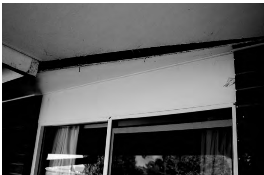
Eave in poor condition.
