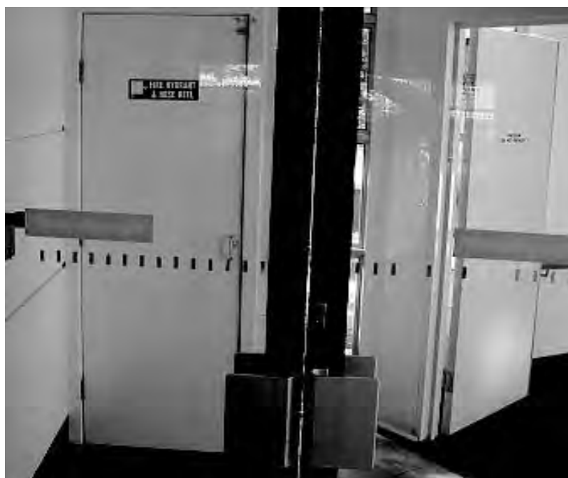
Gap between glass smoke doors reduces their ability to stop the spread of smoke.
