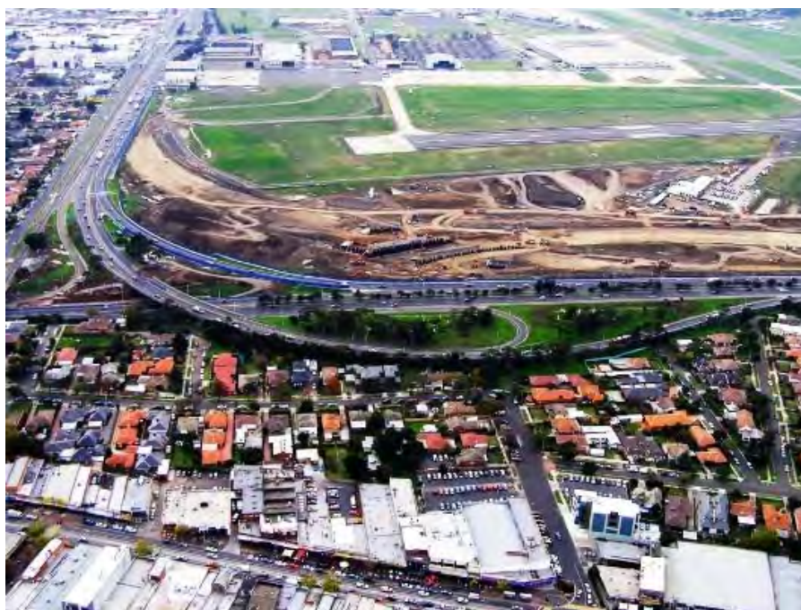
An aerial view of the TCI project at the commencement of works in May 2006.
