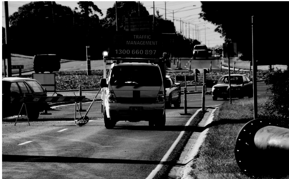
Traffic management is a significant component of external works undertaken by Utility Services.
