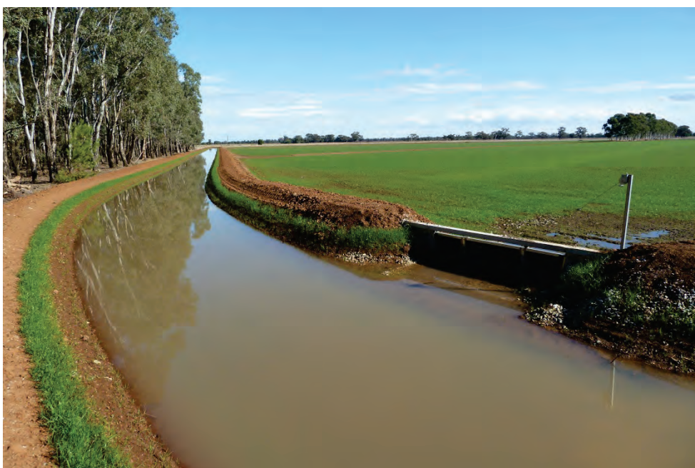
On-farm irrigation upgrade project completed through the Farm Water program. Photograph courtesy of Goulburn Broken CMA.
