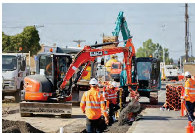
Construction underway to remove the level crossing at North Road in Ormond. Photograph courtesy of the Level Crossing Removal Authority.
